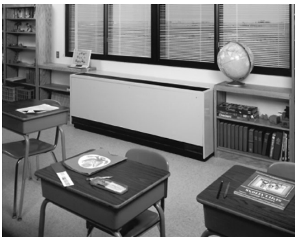
Figure 24. Classroom unit ventilator
